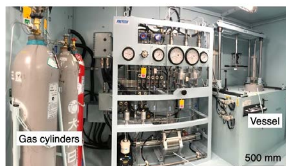
Fig.1. Photograph of the gas loading system at SPring-8.
